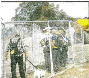
Taking a closer look at the foundations from the temporarily diverted footpath.
